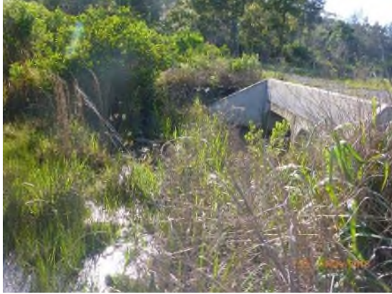
Photograph 4-13 View of the southern extent of the 2 nd order Stream at the culvert on the south-eastern border of the Subject Site
